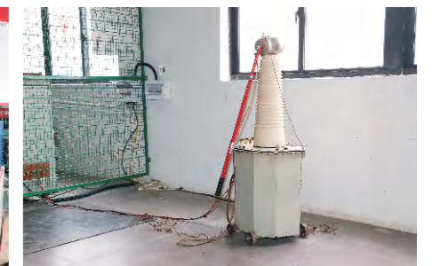
Power frequency withstand voltage test device
